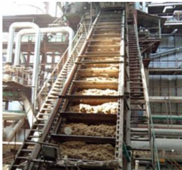
Fig 1. Bagasse carrier Chain conveyor at sugar factory (google image)
